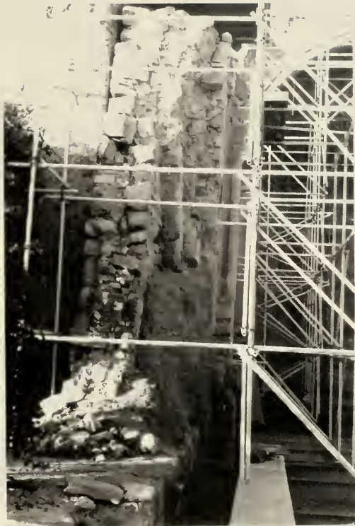
Fig. 5. West wall of nave, Old Stone Church (1994). The load bearing stones are yellow and green sandstone. The core of the wall consists of rubble stone, brick, and lime-based mortar.
